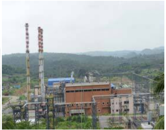
Captive Power Plant
